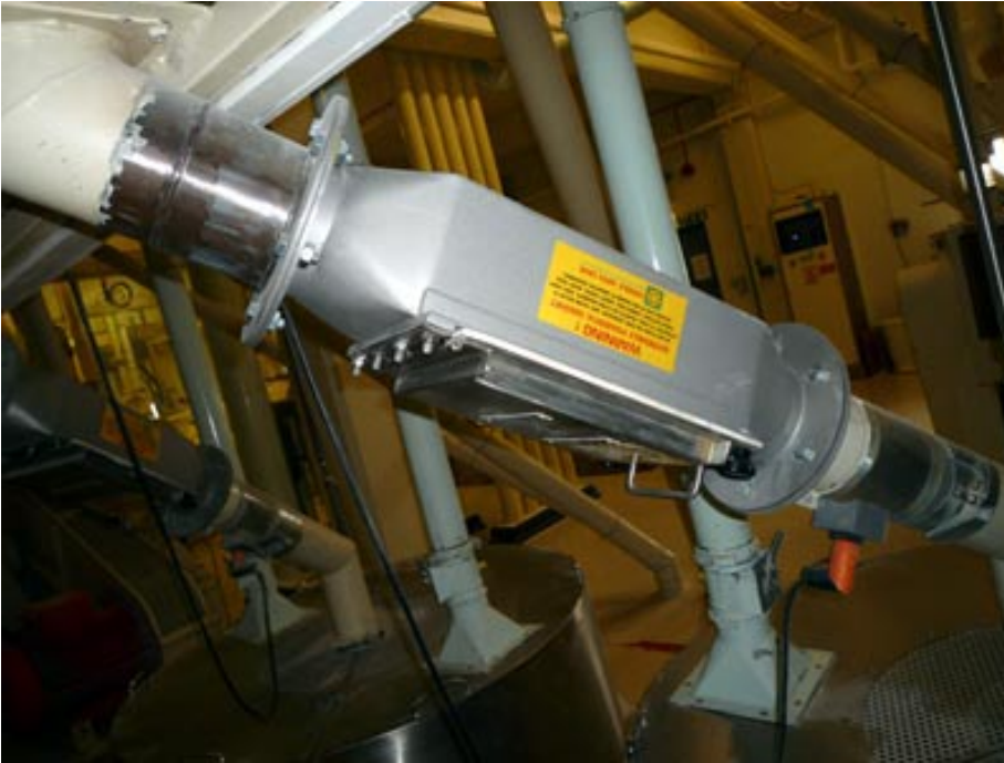
Magnetic plate shown in situ in flour mill
